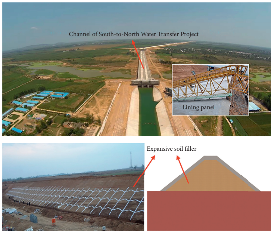
FIGURE 2: Expansive soil filler of high-fill channel in the Nanyang section of the South-to-North Water Transfer Project.
