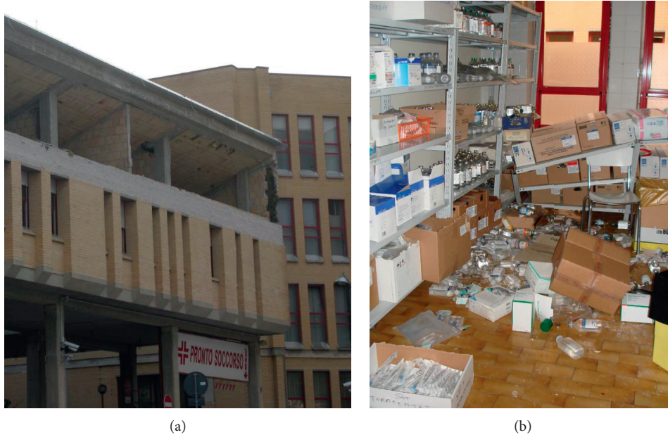
FIGURE 1: Effect of the L'Aquila earthquake (2009) on the Coppito Hospital: (a) falling off the infills on the entry of an emergency room and (b) overturning of shelves in the hospital pharmacy.
