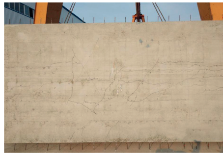
FIGURE 6: The plate cracks of DHB1.
