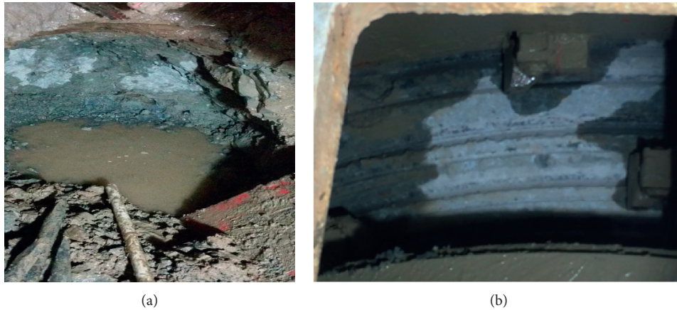
FIGURE 7: Break through plain concrete walls. (a) Drill concrete manually. (b) EPB shield grinding.
