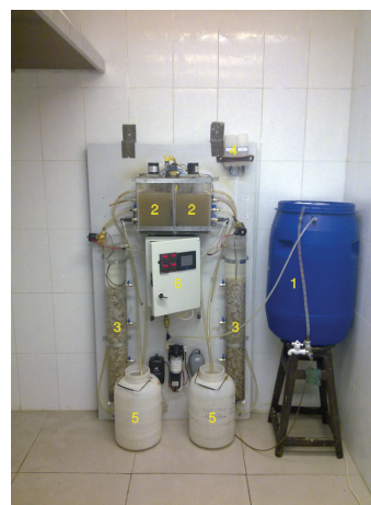
FIGURE 3: Units of reaction pilot: 1—feed tank, 2—aeration tank (SHARON, Single reactor system for High activity Ammonium Removal Over Nitrite), 3—ANAMMOX reactor, 4—pH adjustment tanks, 5—effluent tank, 6—PLC system.
