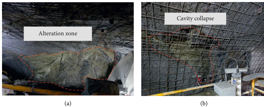
FIGURE 4: Surrounding rock exposed during excavation. (a) Alteration zone with brown muddy at mileage of D1k 225 + 325; (b) cavity collapse at the left arch shoulder at mileage of D1k 225 + 318.
