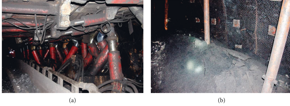
FIGURE 3: In situ coal burst failures in LW5521-20. (a) Collapse of hydraulic supports. (b) Floor heave of the belt roadway.
