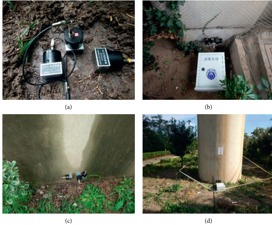
FIGURE 1: Layout of measurement points in the first group of field measurements. (a) GI-1. (b) GI-2. (c) GI-3. (d) GI-4.
