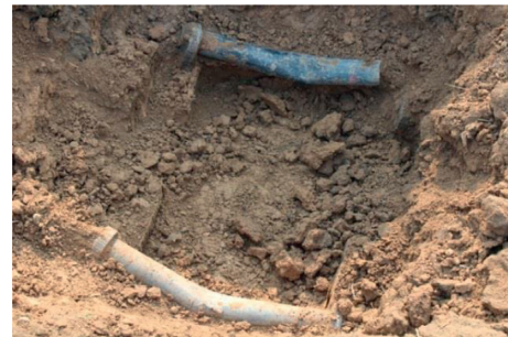
FIGURE 14: Photograph showing one broken end for the standard pipeline.
