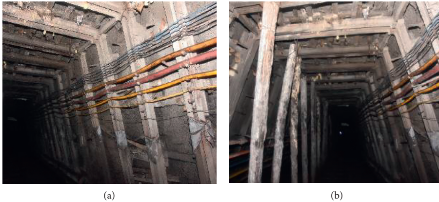
FIGURE 13: Optimization supporting effect of trapezoidal roadway. (a) Middle section. (b) Advanced support section.
