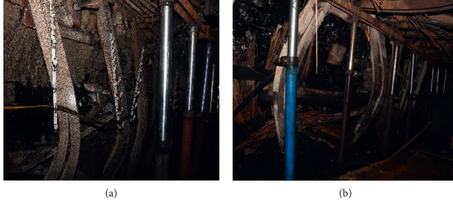
FIGURE 1: The mine pressure of the trapezoidal roadway. (a) The sidewalls of coal pillar heave for 1500 mm. The I-beam bent. (b) The roof declined 500 mm. The floor heaves seriously. The I-beam bent.
