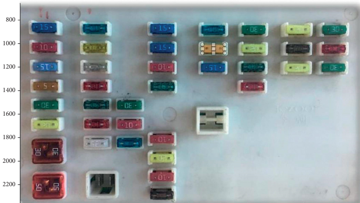
FIGURE 6: The fuse board.
