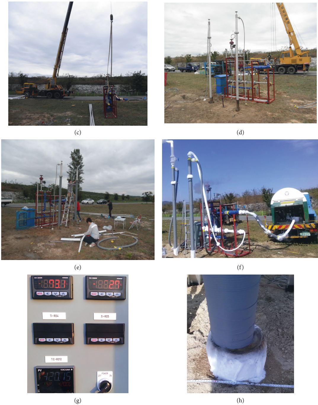
FIGURE 8: Ground freezing system installation procedure. (a) Freezing pipe insertion, (b) inserted freezing pipe, (c) installation of LN 2 supply system, (d) LN 2 supply connected to freezing pipe, (e) pipe insulation, (f) LN 2 supply, (g) automated control panel, and (h) freezing pipe after LN 2 supply.
