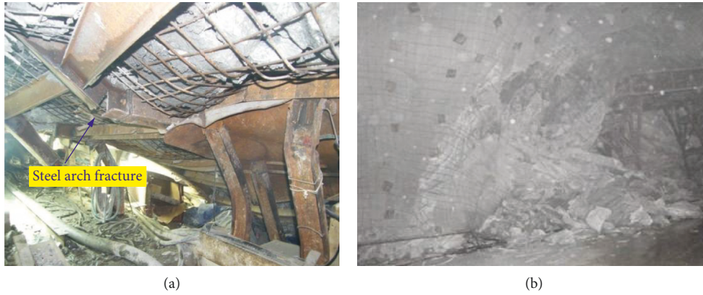
FIGURE 1: Support failure triggers rockburst at the Jinping II Hydropower Station in (a) diversion tunnel #2 and (b) diversion tunnel #4 [6].
