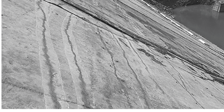
FIGURE 5: Horizontal fractures in the concrete-face slab.
