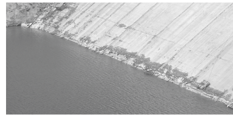
FIGURE 2: Image of slab cracks at Buxi Power Station.
