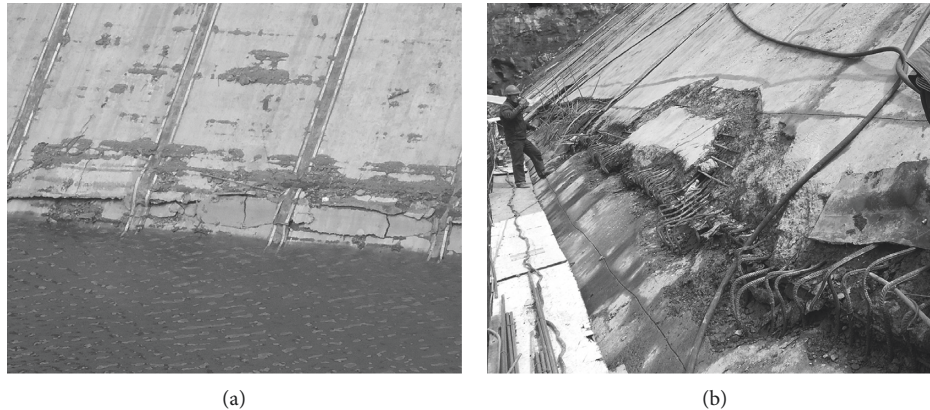
FIGURE 13: Local failure of the face in the phase I portion.
