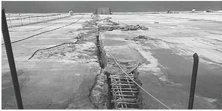
FIGURE 6: Extrusional deformation along the slab joints.
