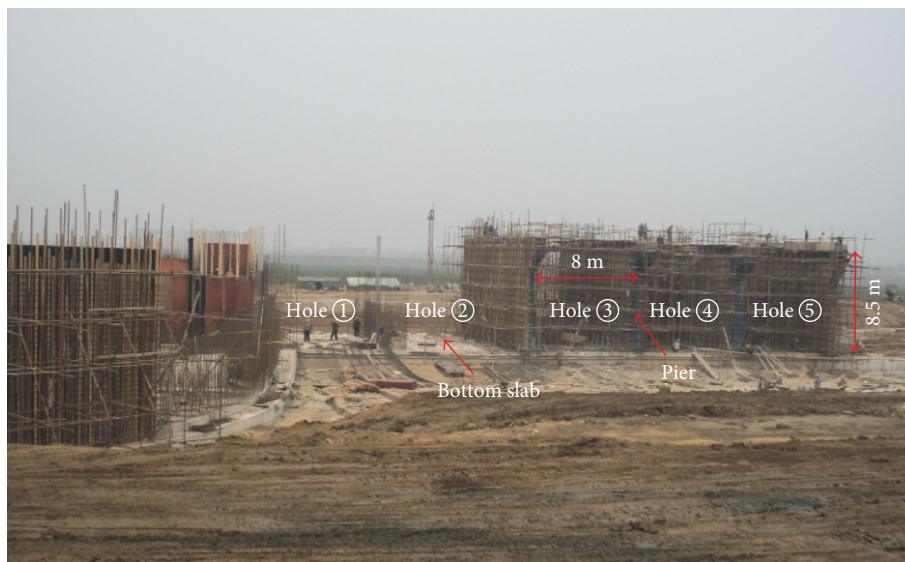
FIGURE 2: A sluice project in the construction period at Huaihe River in China.
