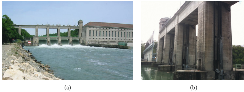
FIGURE 1: (a) General view of the Chancy-Pougny hydropower development scheme [8]. (b) View of the part of the upper dam starting from the cable tower with the three identical piers I, II, and III and their “elephant feet” at the base [10].
