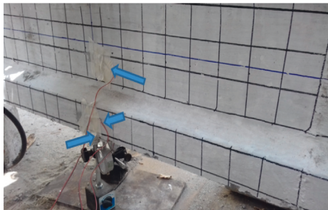
FIGURE 5: Installation of strain and deflection gauges (arrows indicate the position of strain gauges).
