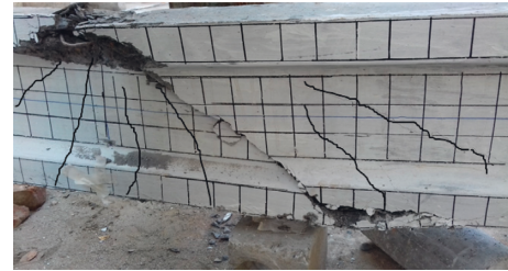
FIGURE 19: Crack patterns of B5-SFRC-1.
