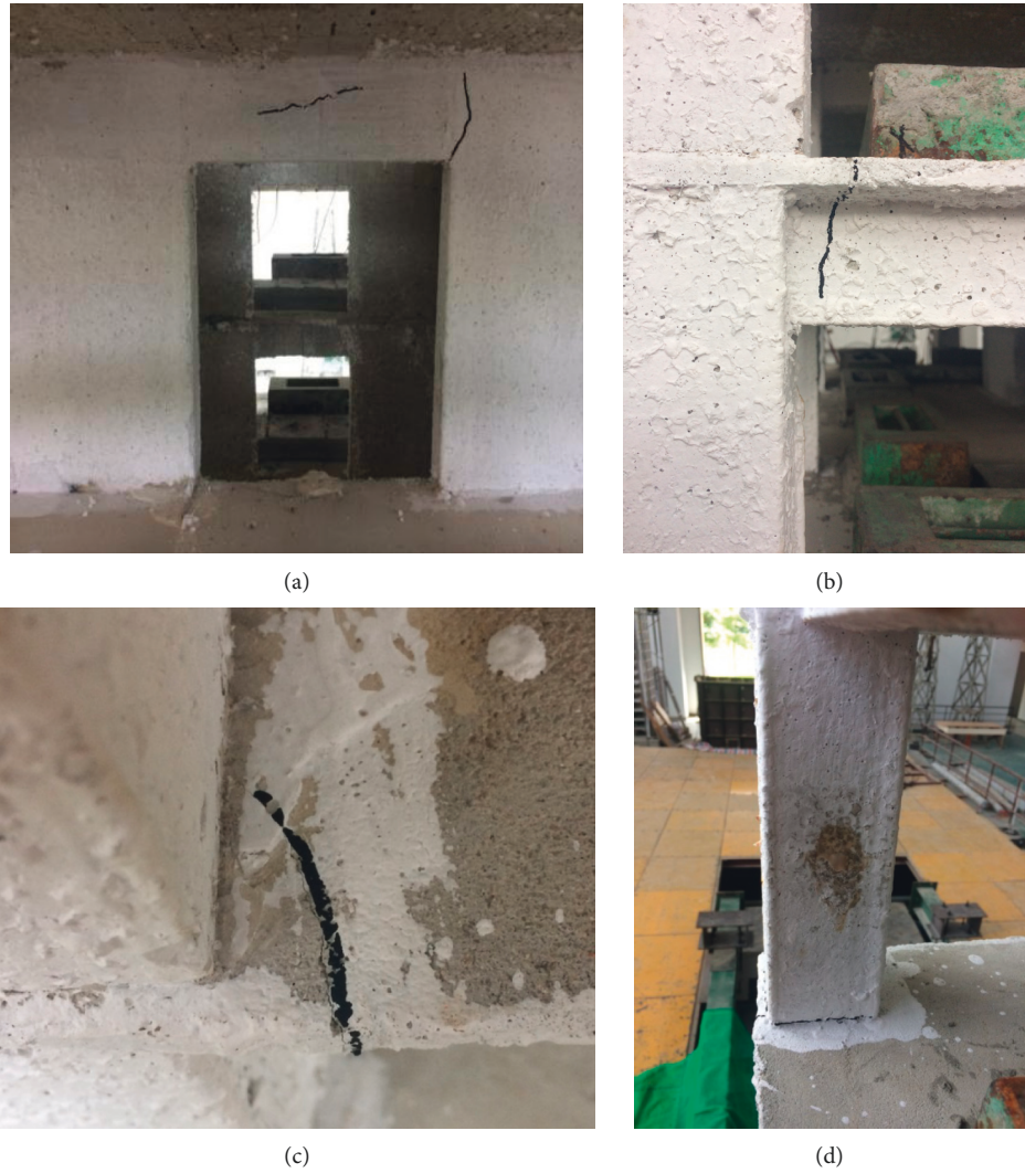
FIGURE 5: Crack of typical components: (a) coupling beam, (b) frame beam, (c) slab of beam end, and (d) intersection of column and beam.
