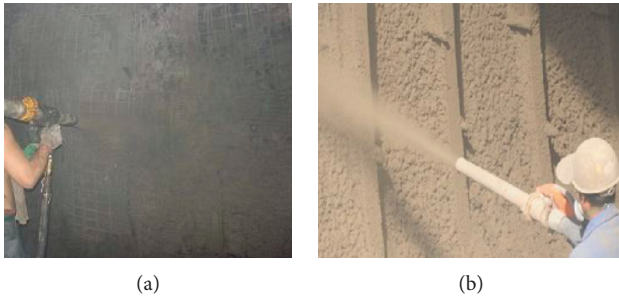
FIGURE 1: Dust production in shotcreting site. (a) Coal mine roadway. (b) Tunnel.
