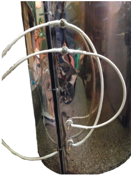
FIGURE 6: Electric heating equipment and interstar connection.
