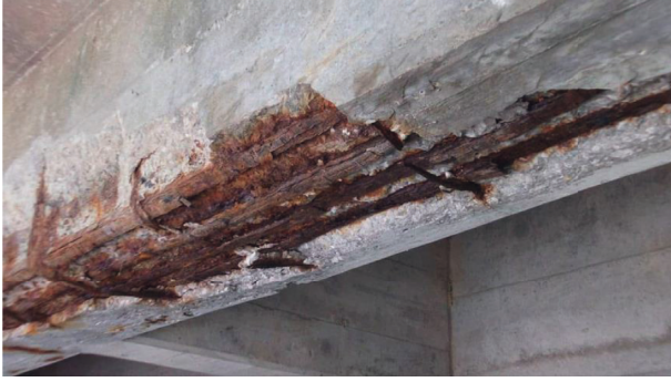
FIGURE 1: Structural performance deterioration of a reinforced concrete (RC) structure caused by reinforcement corrosion [10].
