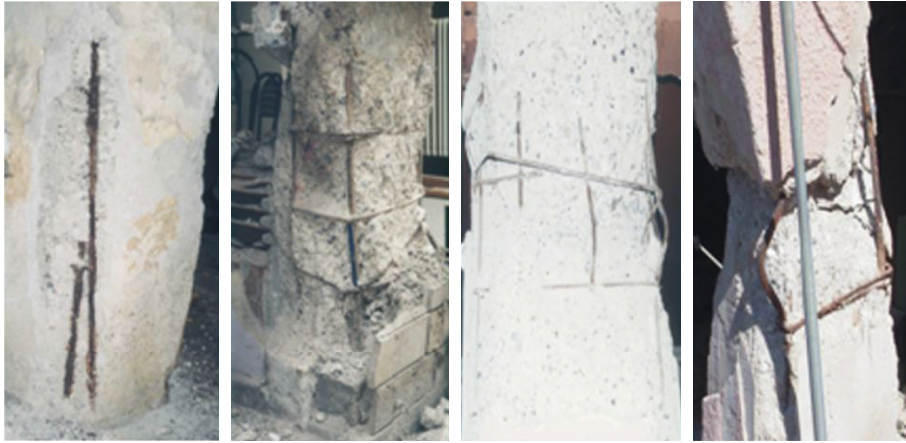
FIGURE 2: Corrosion of RC members damaged during the 1999 Izmit Earthquake in Turkey [7].
