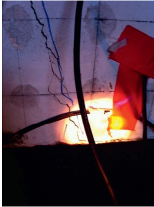
FIGURE 10: Cracks and gap at the connection surface.
