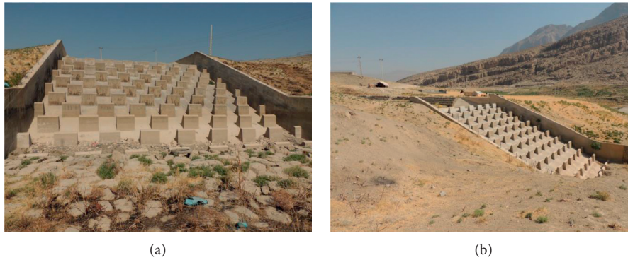
FIGURE 2: The main chute structure with baffle blocks of the irrigation and drainage network on the Doroodzan Dam, Fars province, Iran (the side outlet of Junaki inverted siphon).
