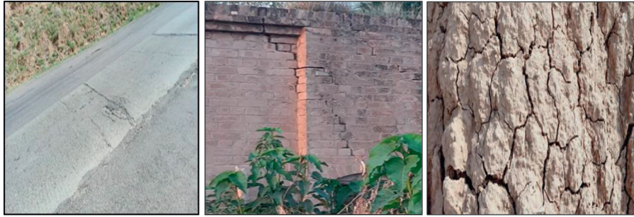
FIGURE 1: Damages due to the presence of expansive soil and desiccation cracks.
