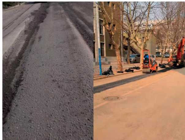
FIGURE 3: Anomalies on the pavement.
