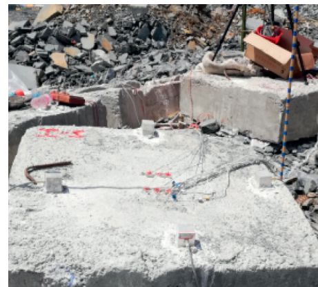
FIGURE 21: Actual layout of blasting vibration sensors.
