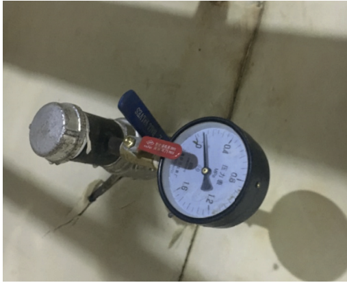
FIGURE 13: Pressure gauge in the pressure relief hole.
