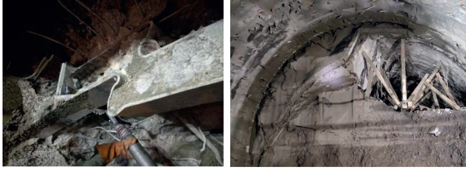
FIGURE 1: Splitting of primary lining and exceeding clearance limit.
