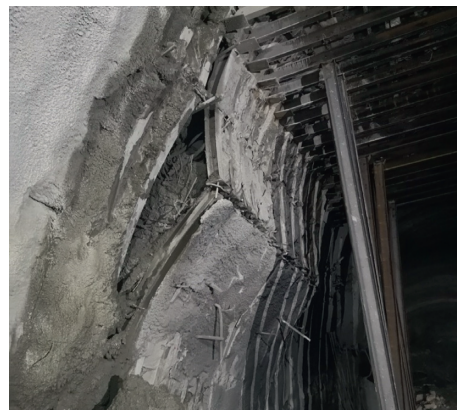
FIGURE 16: Large settlement and convergence at left arch foot of the upper bench.
