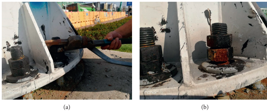
FIGURE 5: Photograph of bolt loosening of the junction of structure A.
