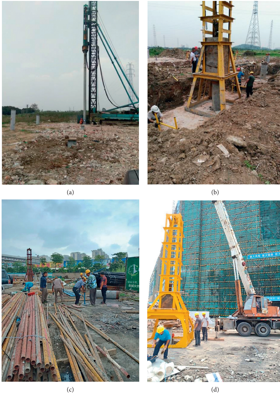
FIGURE 8: Field tests at soft rock bearing stratum (a) and (b) and at hard rock bearing stratum (c) and (d). (a) Pile driving (soft rock bearing stratum). (b) High-strain testing (soft rock bearing stratum). (c) Installation of sliding micrometers (hard rock bearing stratum). (d) High-strain testing (hard rock bearing stratum).
