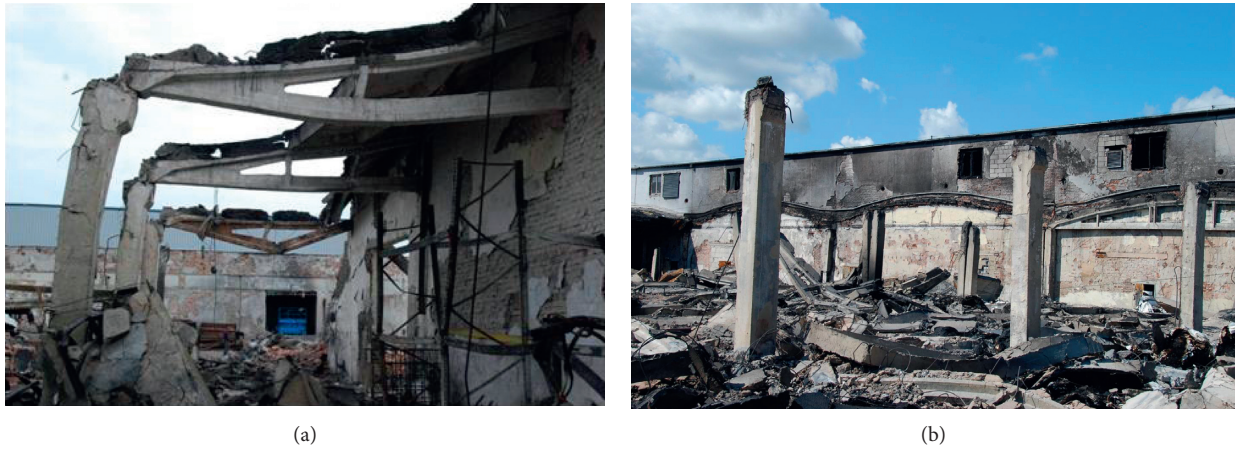
FIGURE 8: Factory condition after the fire: (a) inclined and curved columns and deformed roof girders and (b) collapsed roof [25].
