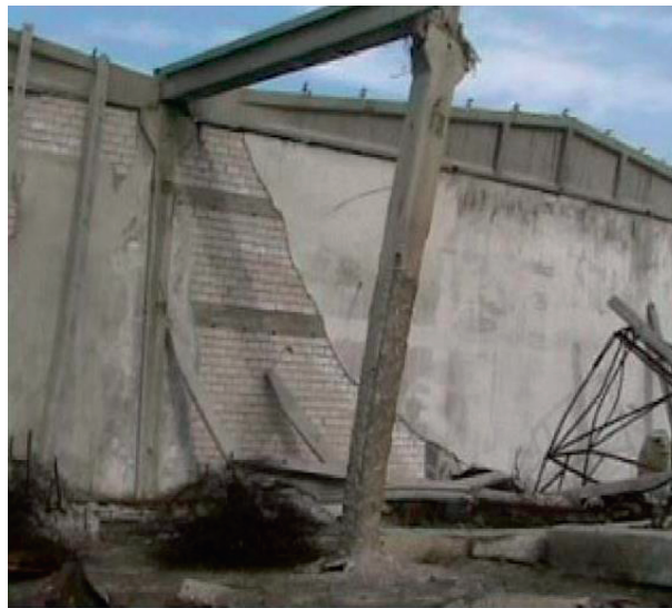
FIGURE 7: General view of the plant after the fire [23].
