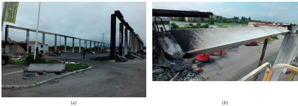
FIGURE 9: General view of the building after the fire: (a) appearance of the objects after the fire and clearing of the ground and (b) beam rotation (tends to decline) [26].
