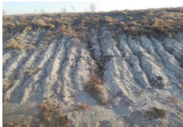
FIGURE 11: Slope erosion of dispersive soil embankment.
