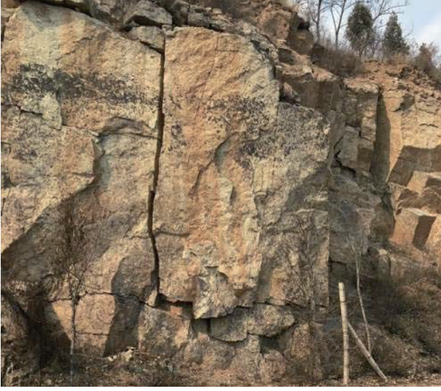
FIGURE 1: Typical hazardous rock block structure.
