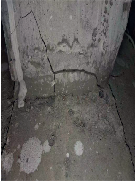
FIGURE 18: Cracks at the bottom of web.
