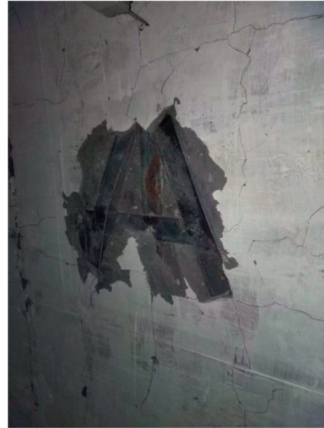
FIGURE 16: Buckling of oblique section steel.
