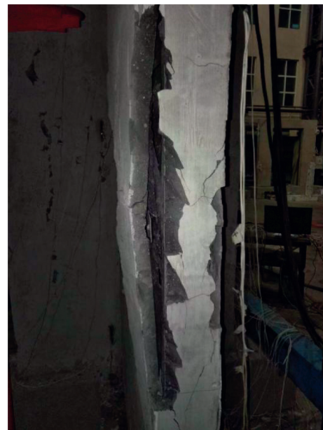
FIGURE 17: Lateral web cracks.
