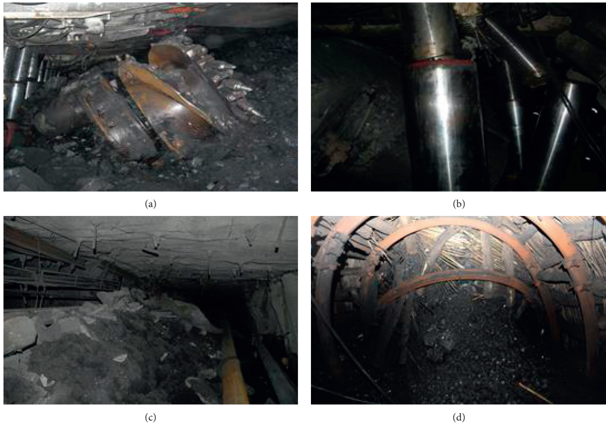
FIGURE 1: Damaged condition of rockburst hazards. (a) Shearer collapsed. (b) Pillar bent. (c) Floor plucked. (d) Broken coal in roadway.
