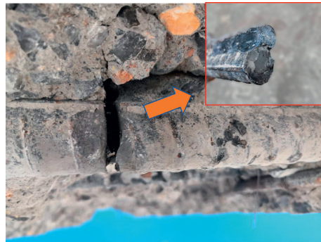
FIGURE 10: Fatigue fracture of steel bar.
