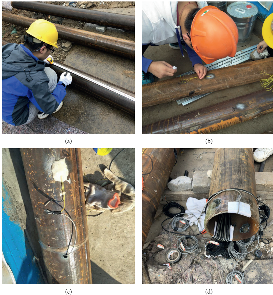
FIGURE 3: Schematic diagram of sensor installation process. (a) Installation location marking. (b) Strain gauge sticking. (c) Strain gauge protection. (d) Data lines fixation.
