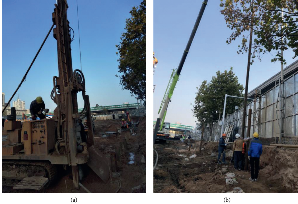
FIGURE 4: Schematic diagram of test pile installation process. (a) Drilling the holes. (b) Test pile lifting.
