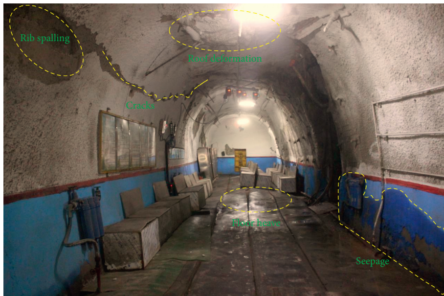
FIGURE 5: The instable conditions of the surrounding rock in the permanent refuge chamber.
