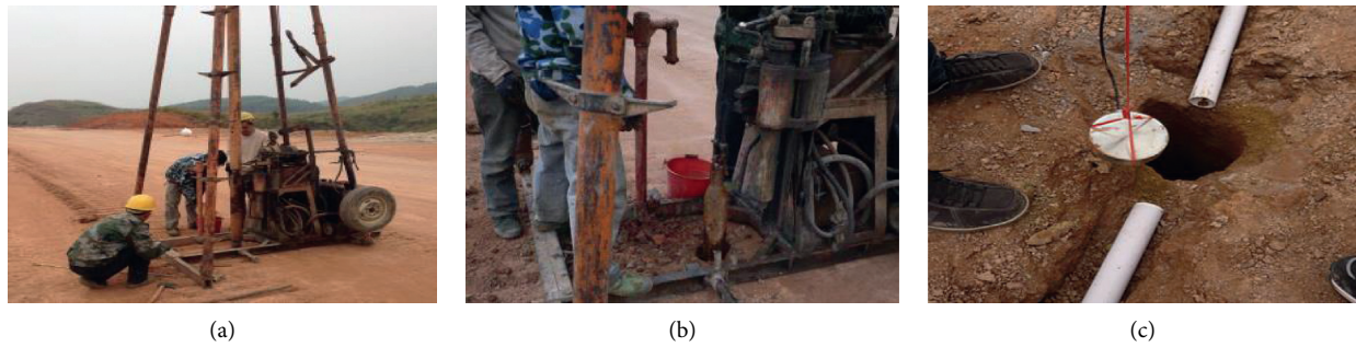
FIGURE 3: Drilling holes for embedding sensors onsite: (a) equipment being in place, (b) impact hole, and (c) placement sensor.
