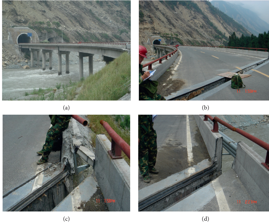
FIGURE 4: Photographs of the Duxiufeng Bridge after the 2008 Wenchuan earthquake. (a) Photographs of the bents. (b) Photographs of the deck. (c) Transverse residual displacement at abutment 0. (d) Transverse residual displacement at bent 3.
