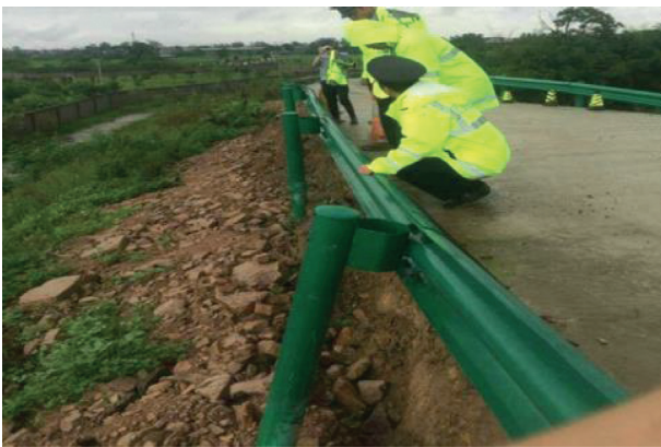
FIGURE 2: Partial subgrade instability (copy from Bing).
