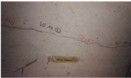
FIGURE 18: Destruction diagram of the right spandrel at the entrance of the tunnel.
