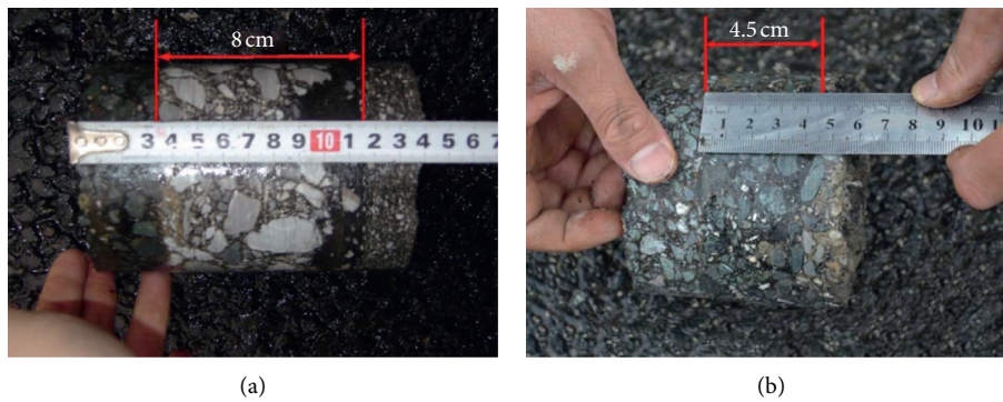
FIGURE 12: Core sample test of asphalt overlay: (a) after one month; (b) after three years.
