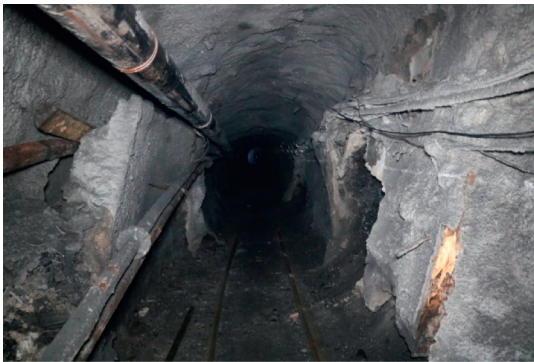
FIGURE 2: Spalling rib forms of surrounding rocks in deep roadways.
