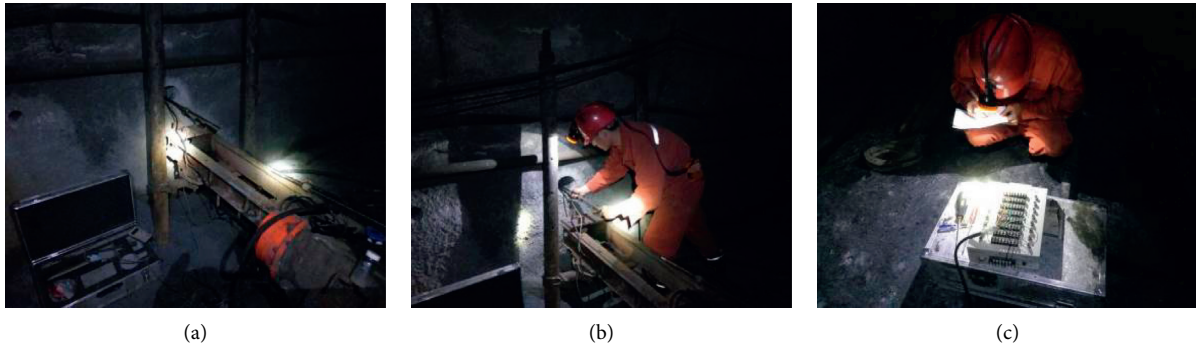
FIGURE 2: Filed test process. (a) Drilling construction. (b) Stress gauge installation. (c) Data collection.
