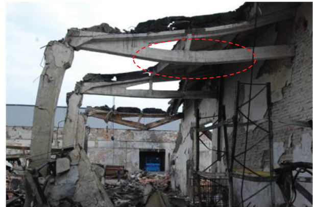
FIGURE 11: Deformation of the centre of the RC girders in a real fire incident [74].
