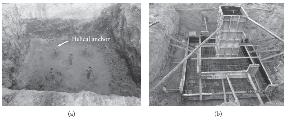
FIGURE 4: Photo of a composite foundation prior to concrete placement: (a) installed helical anchors and (b) the footing with reinforcement and supporting wall framework.
