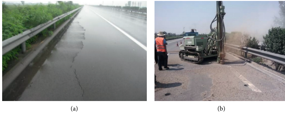
FIGURE 1: Longitudinal cracks and drilling rig operation at K555 + 800 (in Yinchuan direction).
