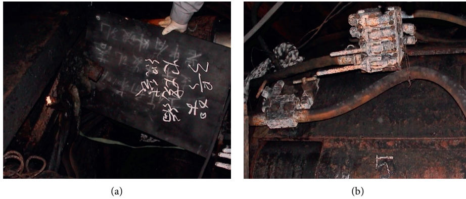
FIGURE 9: Main damage evidence in field investigation.
